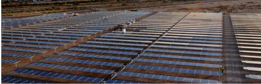
-5 MW PV farm 5
